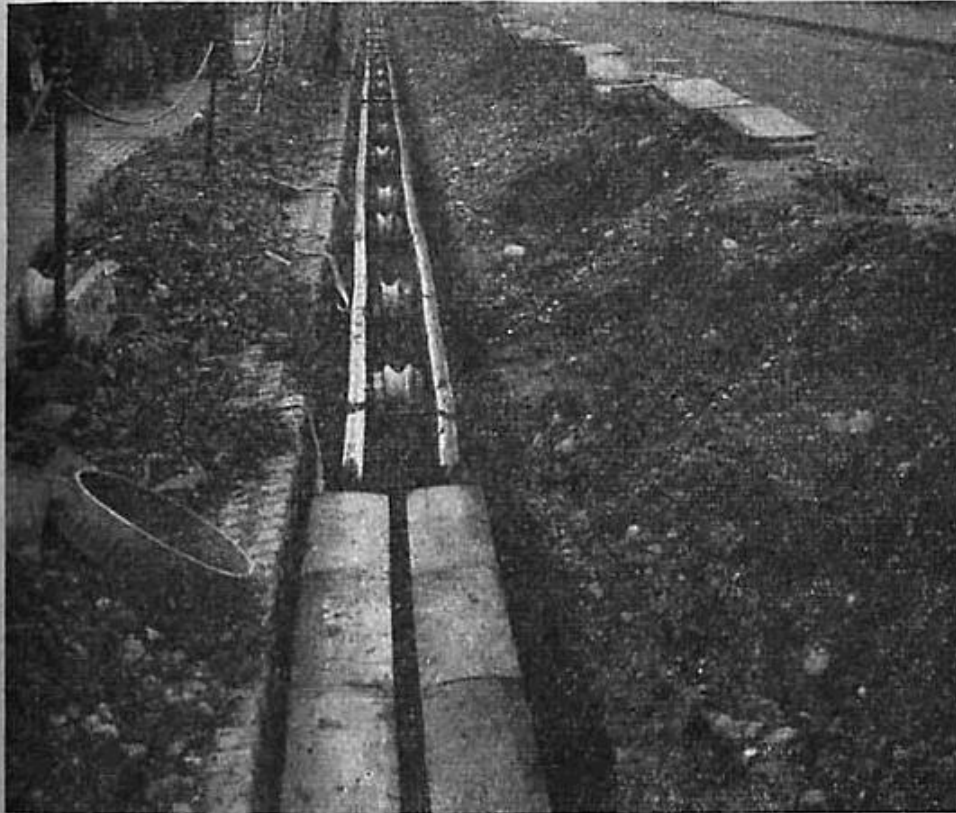
FIG. 79. CABLES IN TRENCH PROTECTED BY CONCRETE COVERS
